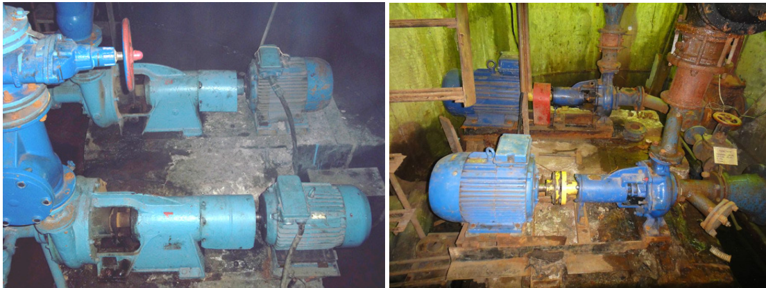
Fig. 1. Appearance of pumps mounted at sewage pumping stations in small towns and villages
